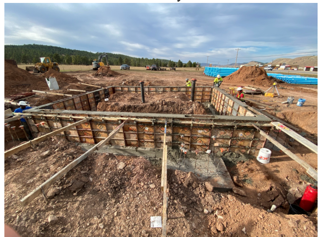
New $1.24M wellhouse under construction for Black Hawk Water User District. Wellhouse will pump & treat well water to future 500K gallon concrete tank.
