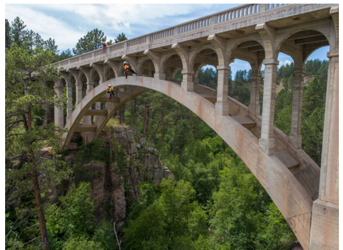
Wind Cave Bridge Inspection completed on July 30-31, 2020 by HDR. The in-depth inspection is a part of the much larger rehabilitation effort for the bridge.
