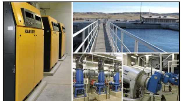
South Dakota Ellsworth Development Authority Wastewater Treatment Facility. Submitted by SEH
